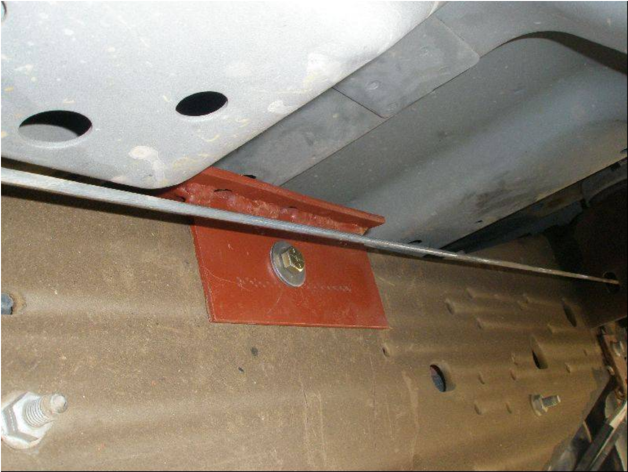
Figure 6. The filter head mount outside the frame. The two Grade eight 5/16" bolts (one unseen in this pic) use existing frame holes, eliminating the need to drill the frame. Simple 3/16" x 2" stock welded to scrap 3/16" x 2" x 4" angle.
